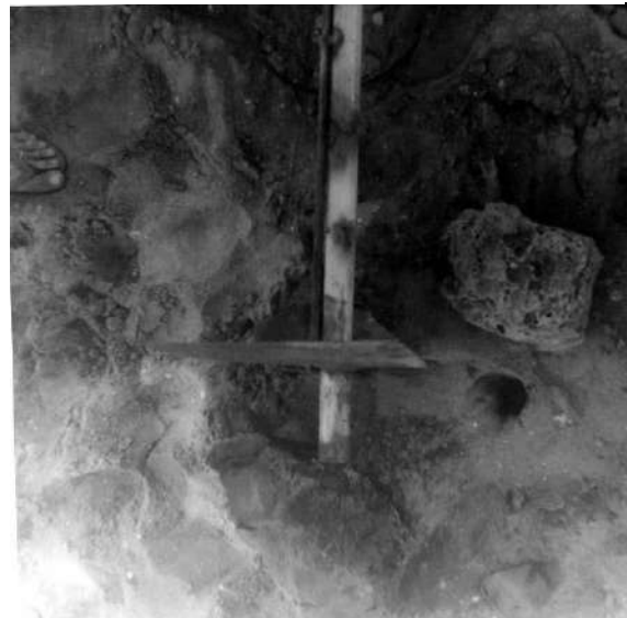
B-2 punched through steel pad – note hole in ground to right
